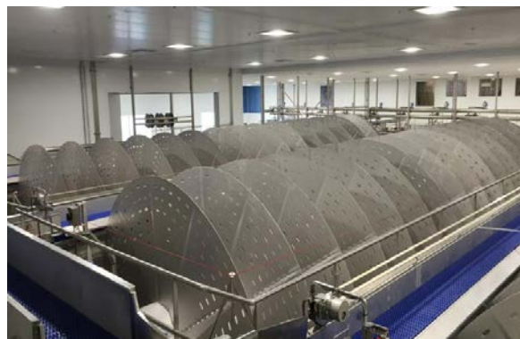
Figure 2: Chilling tank at salmon slaughter plant
