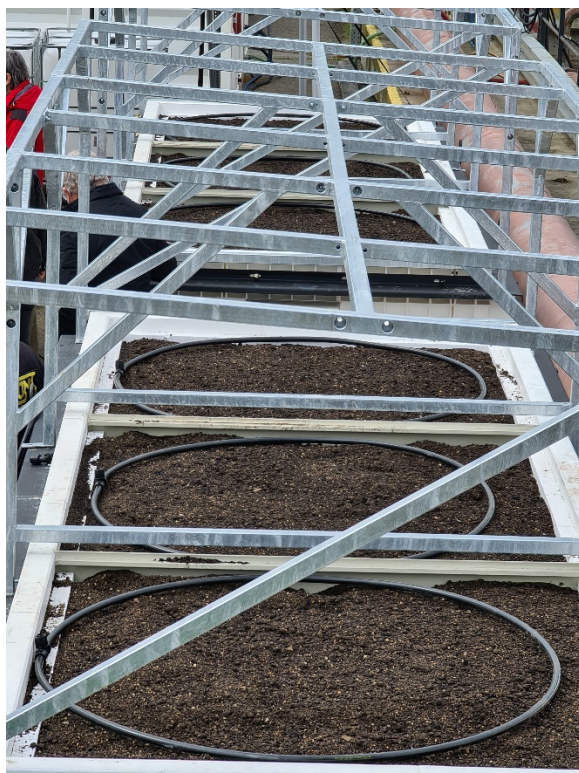
Figure 10: Irrigation system and support structure for roof over the boxes
