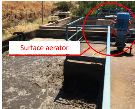
Figure 7: Existing surface aerator at Corleone WWTP
