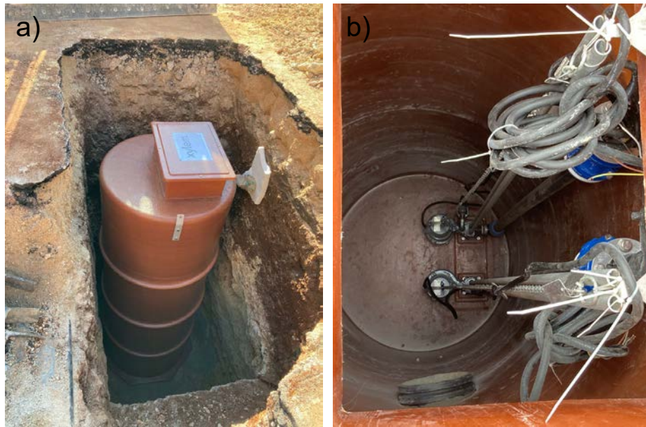
Figure 21: Installed Fiberglass polyester tank (a) and pumping station (b) of the real wastewater
