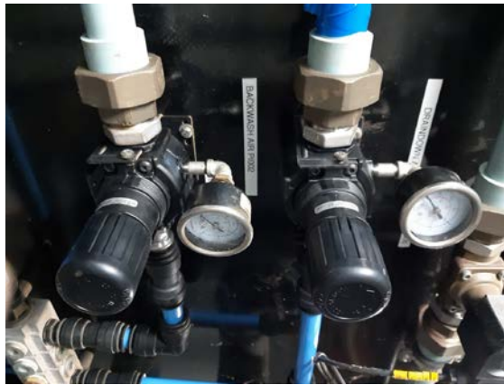
Figure 5: New pressure regulator of the UF modules
