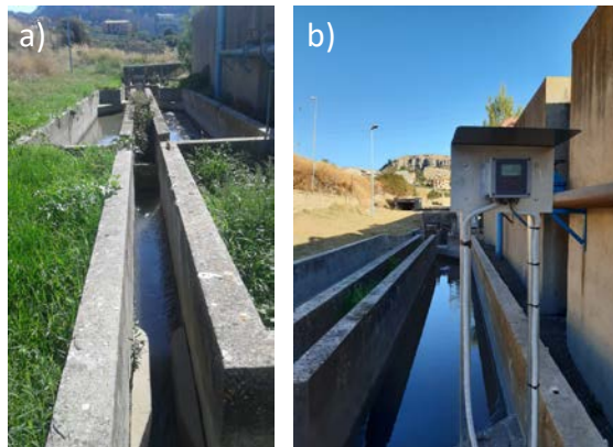
Figure 1: Before (a) and after (b) flow meter installation at the plant inlet
