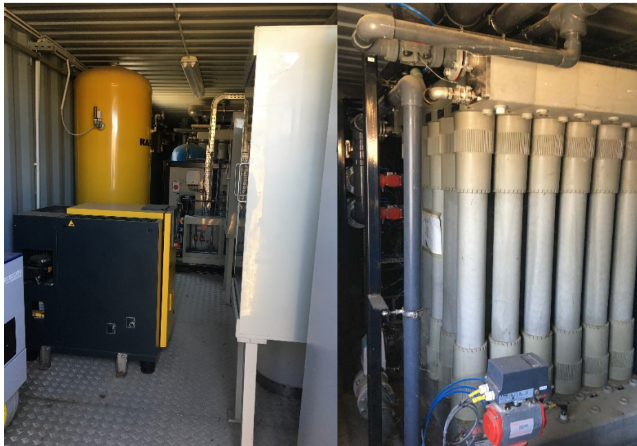
Figure 6: View of the ultrafiltration membrane treatment system
