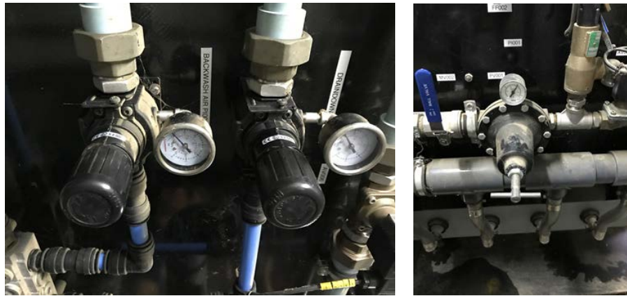
Figure 3: Pressure regulator of the UF modules before maintenance
