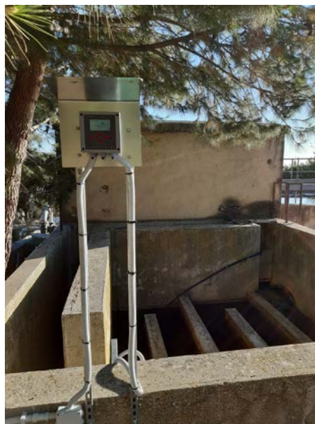
Figure 2: Flow meter installation at the plant outlet
