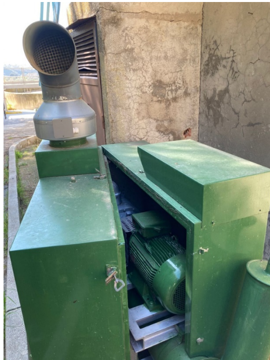
Figure 10: View of the blower of the new aeration system
