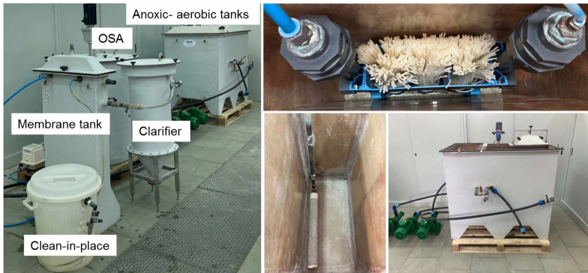
Figure 24: Panoramic view and details of the pilot plant for wastewater treatment
