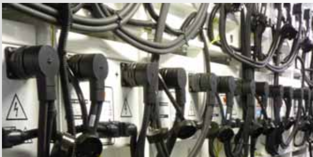
Power shaving/ spinning reserve batterier Brenselselle
