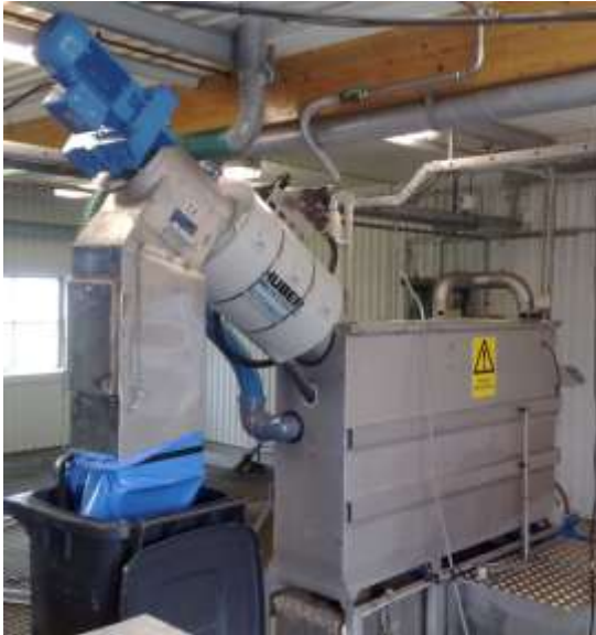
Ro9 i tank
