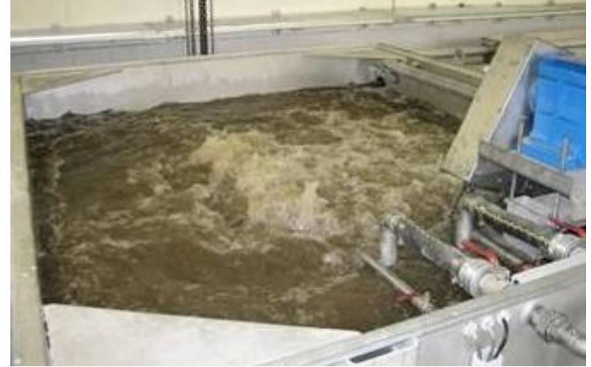
Filtration tank, HUBER BioMem® plant
