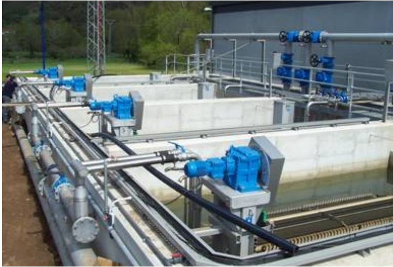
4 VRM® 30/448-Units in filtration chambers
