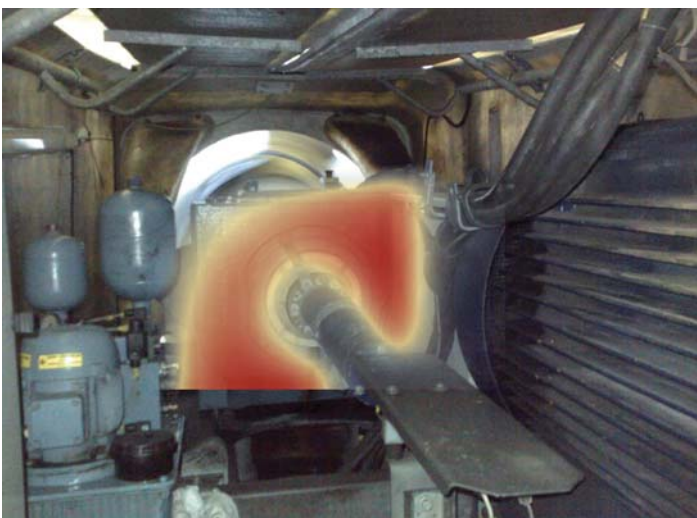
Screenshot of collected sensor information from a pilot installation at VIVA test center
