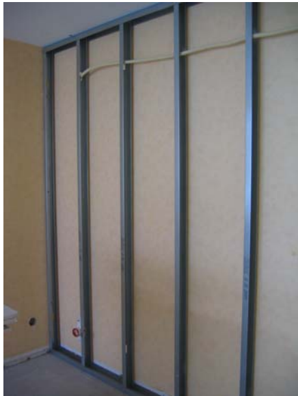
Figure 7 Sound insulation of inner wall
