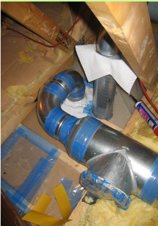
Sleeves (white) are used for tightening between the vapour barrier and the ventilation ducts penetrating the attic floor before insulation is added. (The sleeve to the right is not mounted yet)
