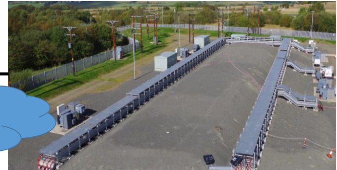
PNDC: Electrical network & network assets
