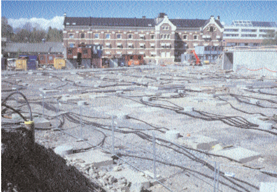
The wellfield for the Nydalen GSHP in Oslo, Norway; the station will supply several buildings
