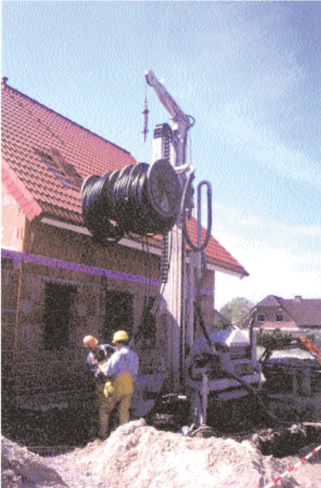
Installation of borehole heat exchanger at a small house in Bielefeld, Germany, using a small, powerful Rotomax drilling rig
