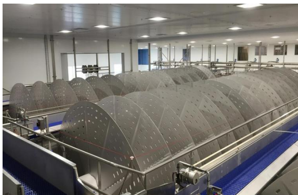
Figure 2: Chilling tank at salmon slaughter plant
