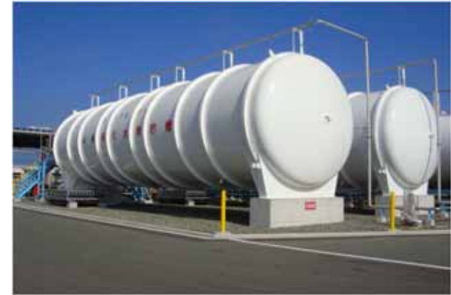
Liquefied hydrogen storage tank
