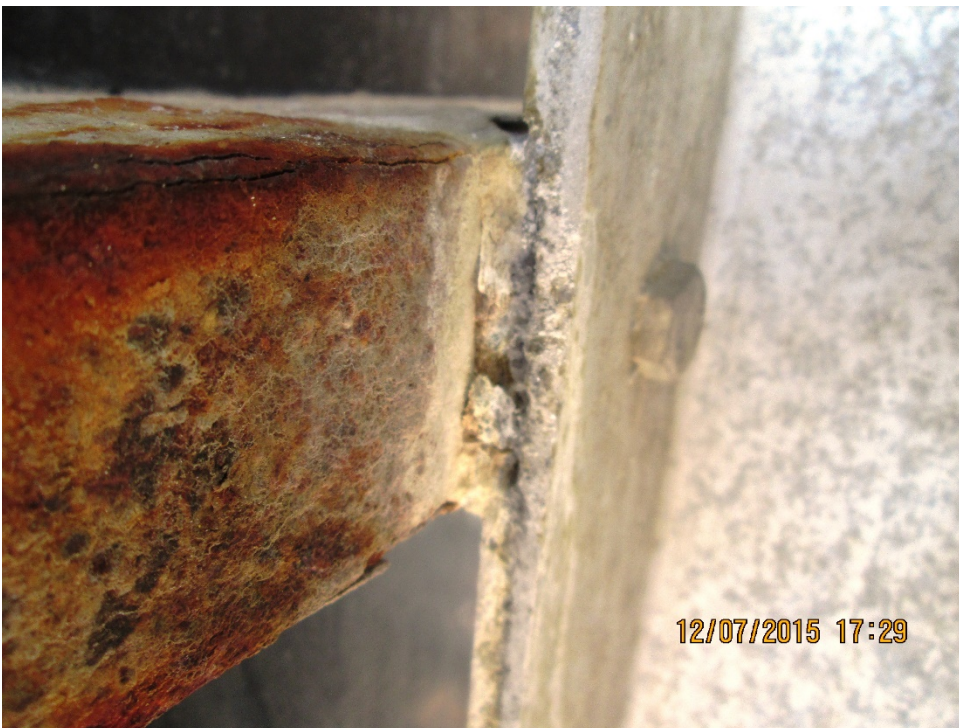
Figure 7. Galvanic corrosion at a connection between an aluminum signage on the right and a steel structure on the left connected by a stainless steel bolt.
