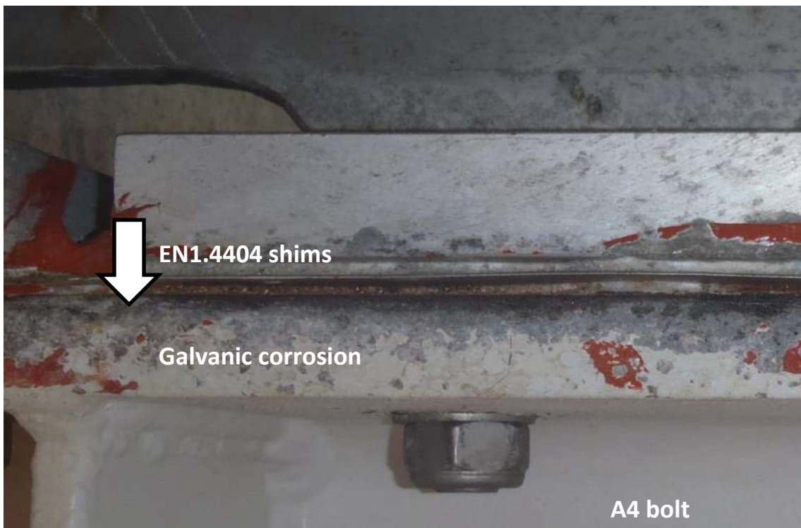
Figure 5. Galvanic corrosion on aluminium around EN1.4404 shims in a bolted joint [25].
