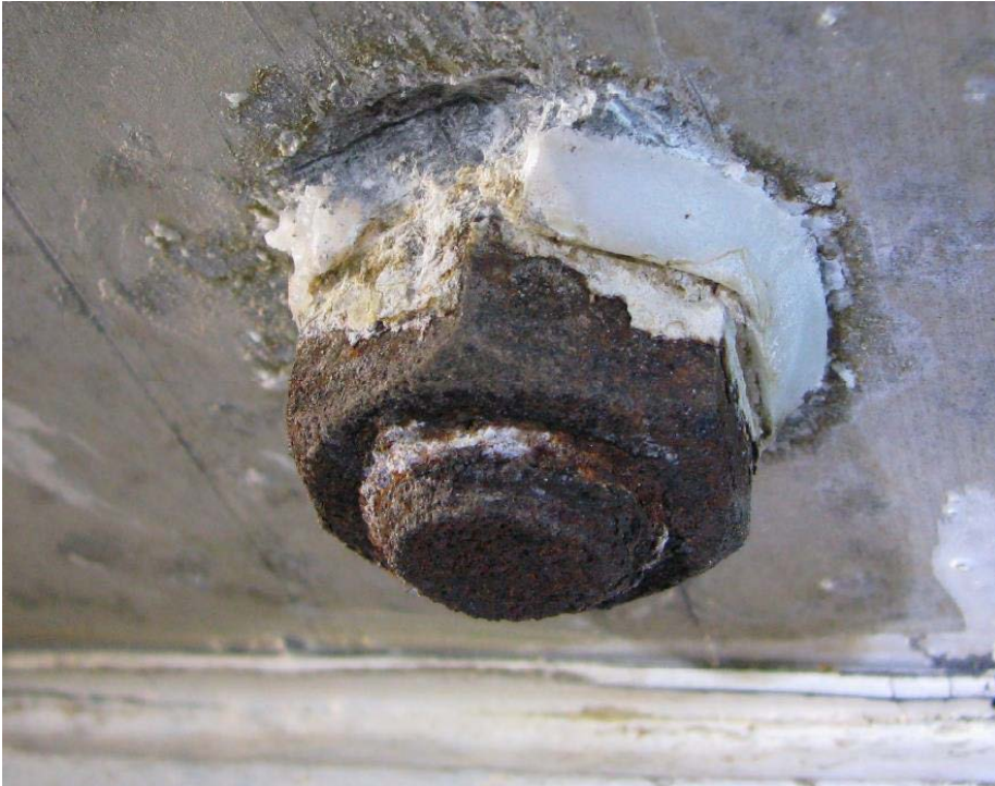
Figure 6. Galvanic corrosion around galvanized bolt with nylon sleeve. The zinc has corroded away and the nylon sleeve has degraded, so that the bolt steel is in direct contact with the aluminium and causes galvanic corrosion [25].
