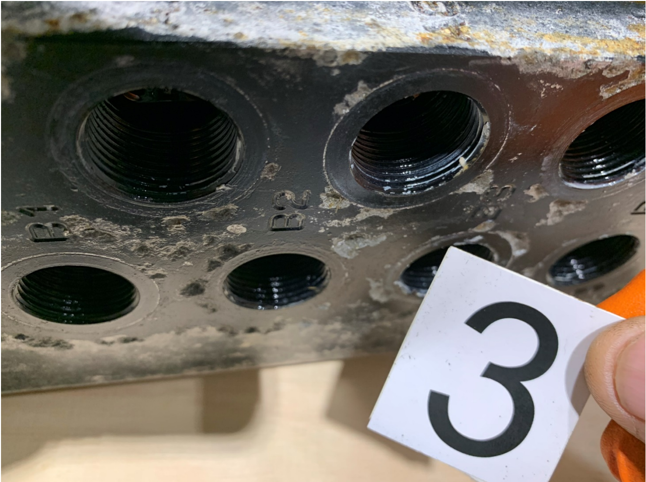
Figure 14. Galvanic corrosion and alkaline etching around stainless steel parts screwed into anodized aluminium
