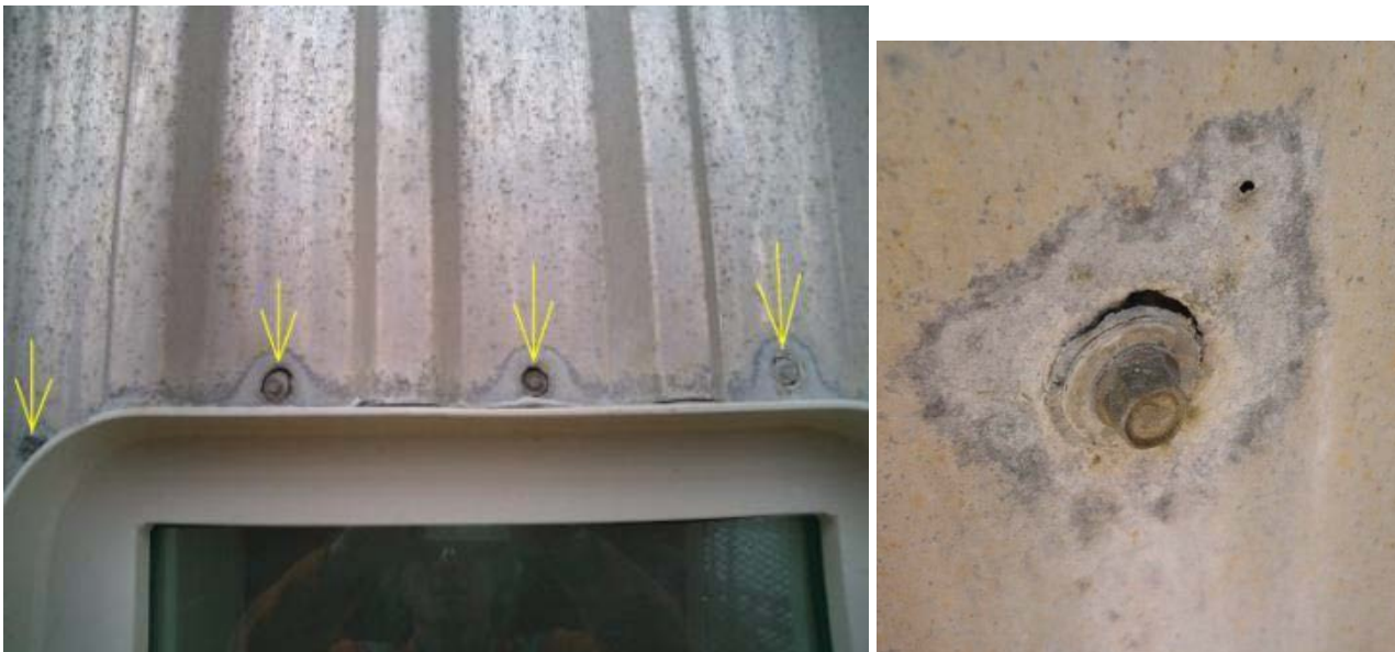
Figure 4. Galvanic corrosion on aluminium around stainless steel bolts (A4). Close-up to the right [25].
