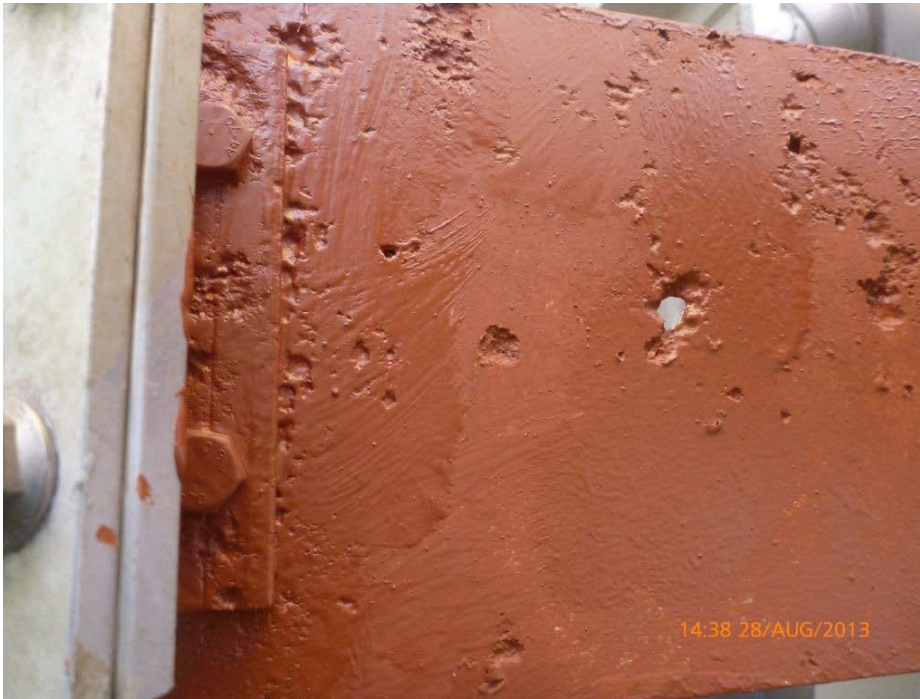
Figure 8. Pitting corrosion under passive fire protection (PFP). The PFB absorbed water and the aluminium surface was constantly wet, resulting in severe pitting corrosion [25].
