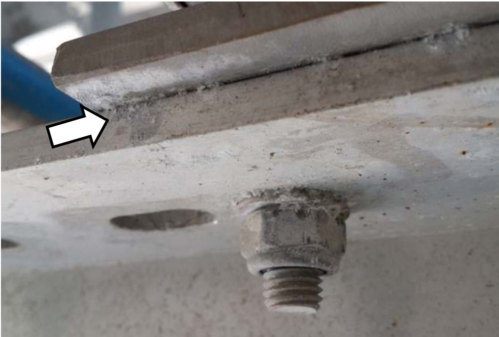
Figure 9. Crevice corrosion in Al-Al bolted joint, and galvanic corrosion around A4 bolt [25].
