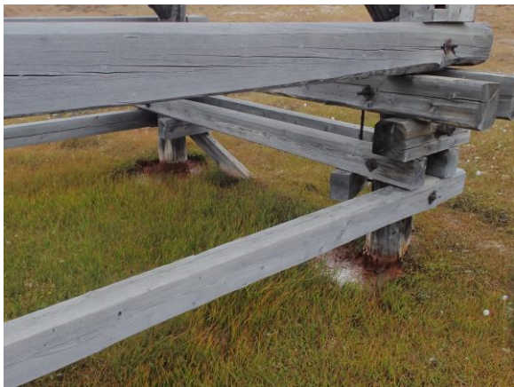
Line 6, Bukk 27 (pictures 27_5 and 27_7) – changes in vegetation and depressions around foundations, spin-off effect – ponding of water
