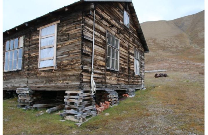
Boligbrakke G in Hiorthhamn, Svalbard (summer 2021) with temporal foundation solution as described in (Boro and Flyen, 2021). This temporal solution is in place for 18 years as for 2021.
