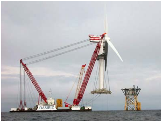
Figure 32: Transport and installation of a wind turbine constructed onshore at Beatrice (Source: www.scaldis-smc.com )
