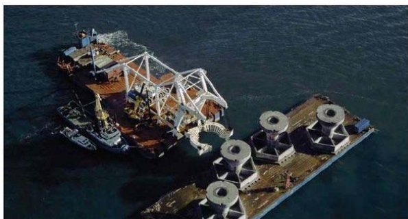
Figure 29: Installation of the gravity base structure at the Nysted wind farm (Source: Danish Energy Authority)
