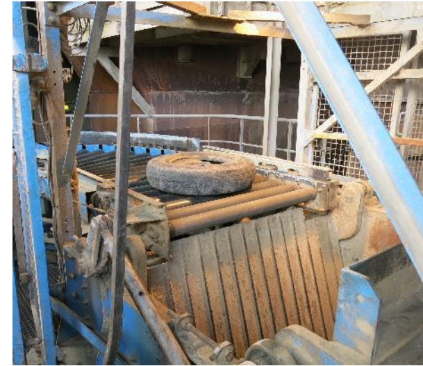
Calciner fuel feed
