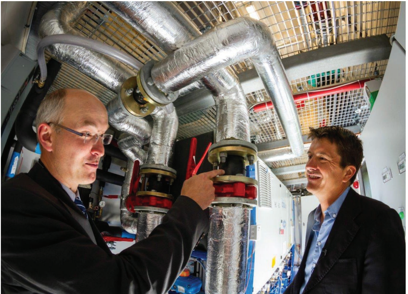
Senior scientist Armin Hafner and Rema managing director Ole Robert Reitan in the supermarket's refrigeration-machinery space.
